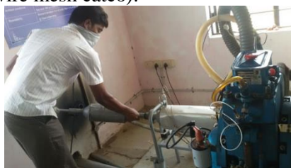
Figure.9. Installation of non-noble based catalytic converter on DI Diesel engine
